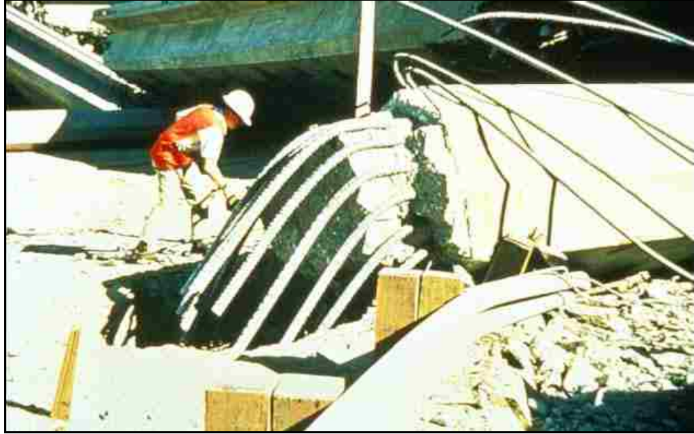
Figure 2.8 Pullout failure, 1971 San Fernando earthquake (Caltrans, 2003)
